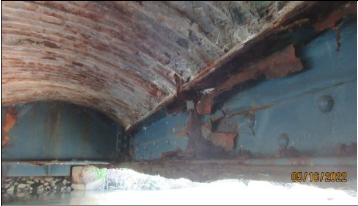
Underside of Deck Condition and Steel Girder Deterioration
