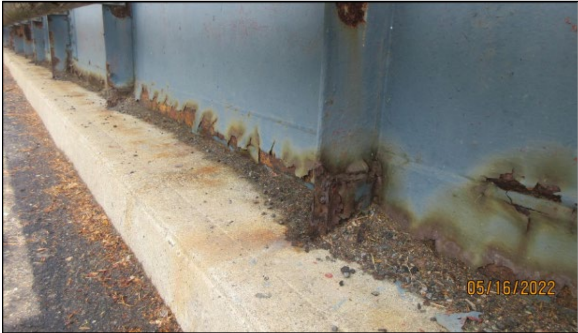
Steel Through-Girder Deterioration Along Curb
