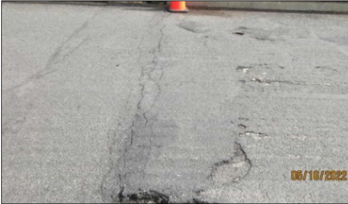
Transverse Cracking and Potholes along Deck Surface
