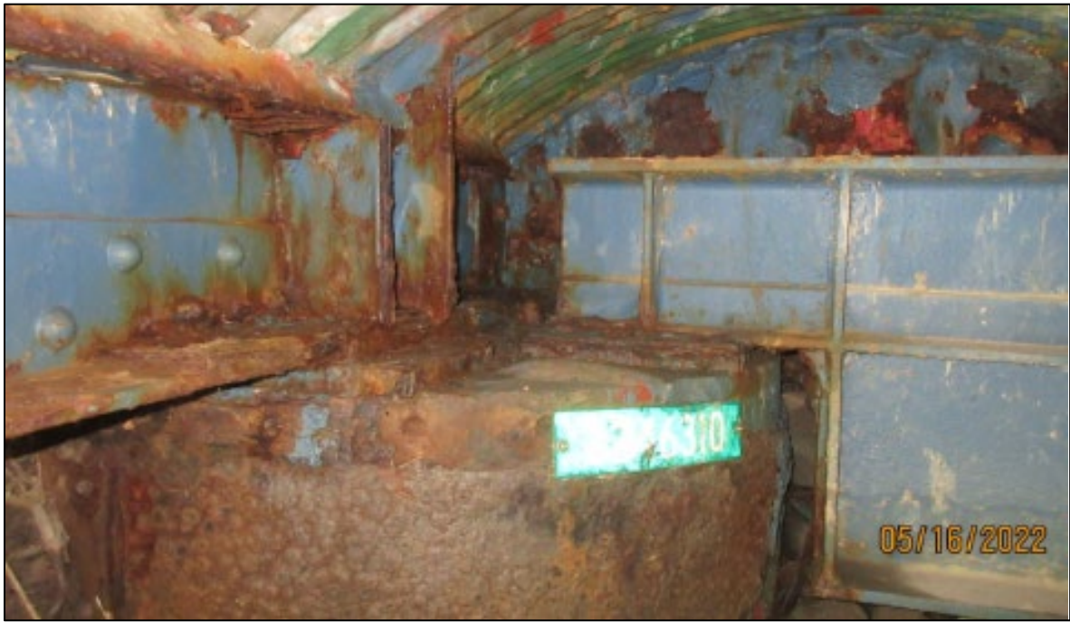
Bridge Bearing and Steel Framing Deterioration
