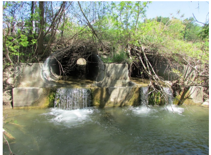
Figure 1: Culverts such as this one constrict the natural flow of the stream and contain no natural streambed substrate. Perched culverts such as this one fragment stream habitats.
